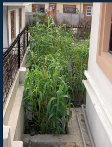
Reed bed for greywater treatment — 4.8 m 2
