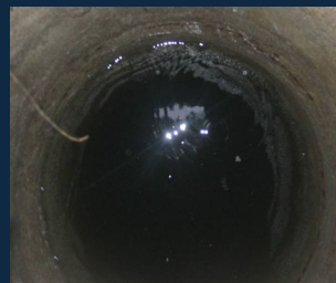
Underground water collection tank
