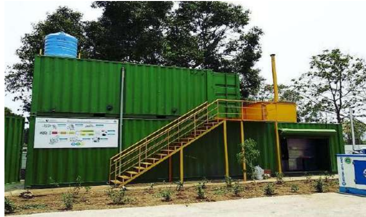
Wai FSTP (Pyrolysis Technology)
