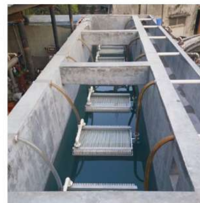
FIGURE 06: View into MBR system with membrane modules. Source: Chem Limited.
