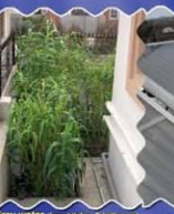
Grey water treatment system (Constructed Wetland) Area: 5 Sq.m.
