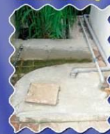
Ground water recharge through dugwell
