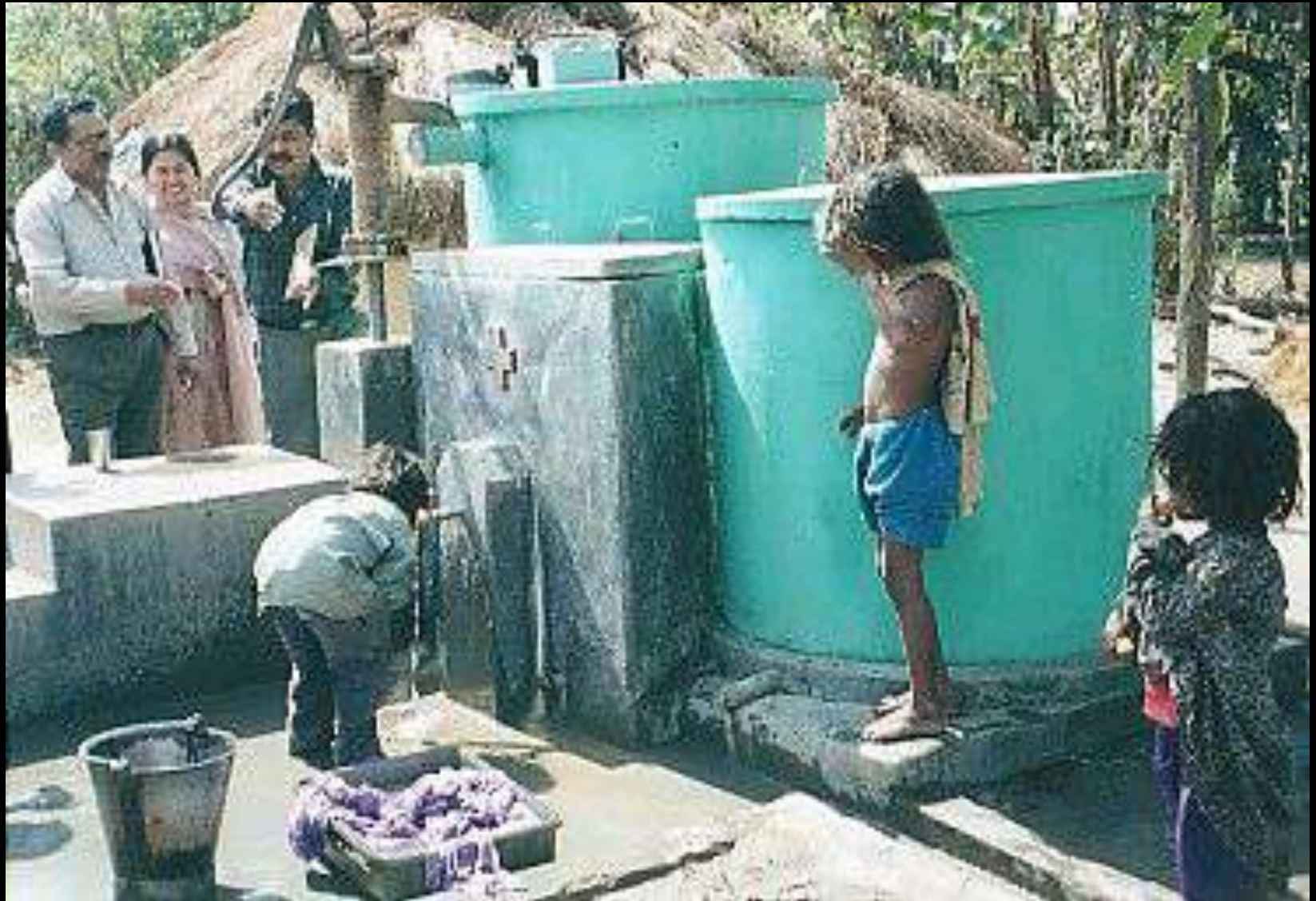
Arsenic- Iron Removal Plant in Badera VDC in Nawalparasi
