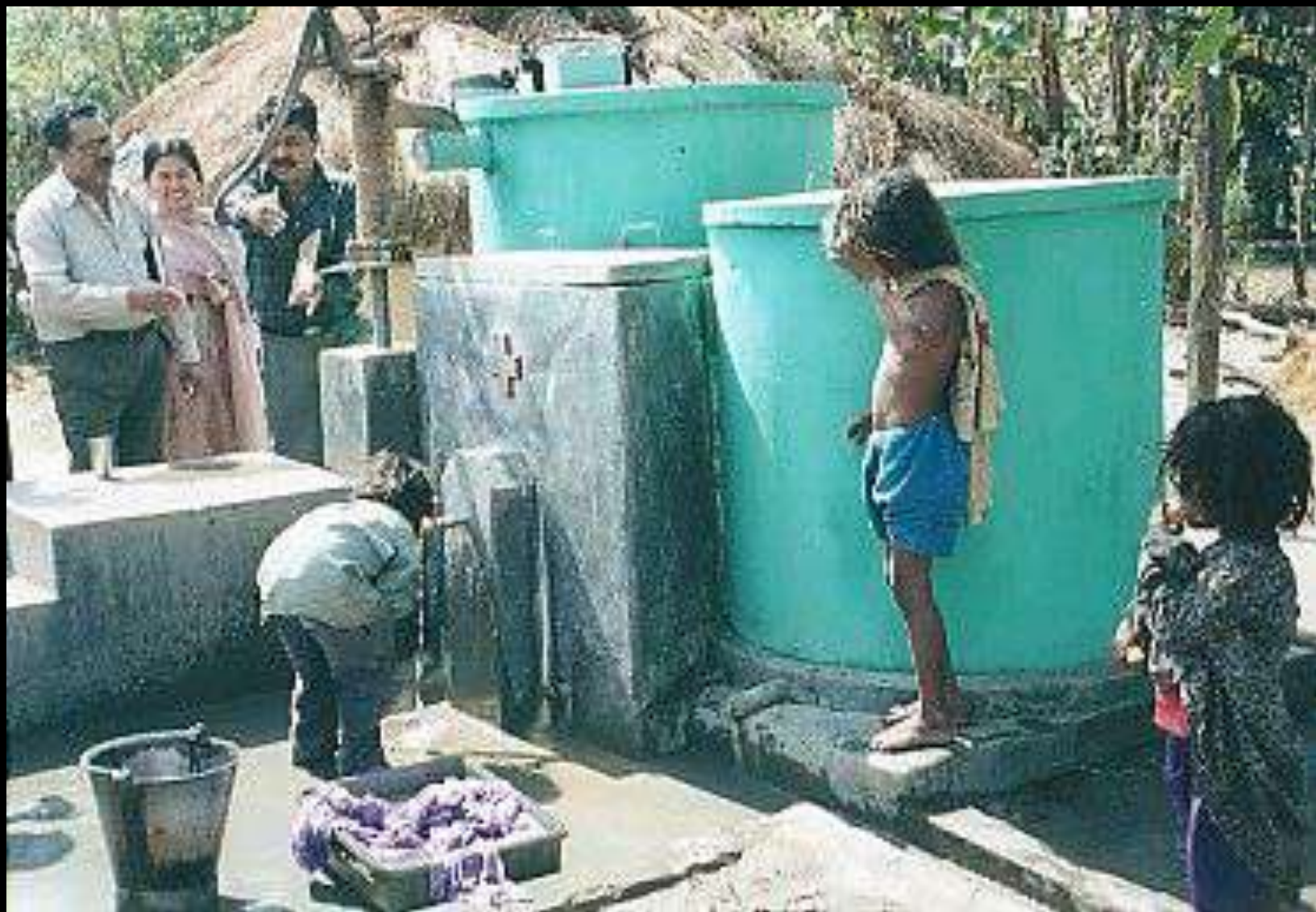
Arsenic- Iron Removal Plant in Badera VDC in Nawalparasi
